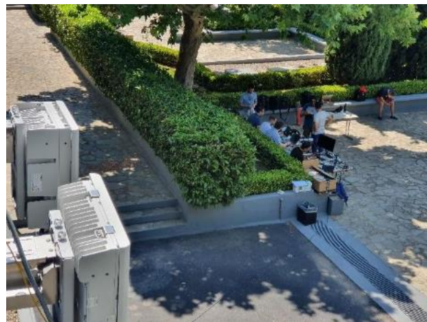
Figure 13 - Ericsson Radio 4408 n78R equipment at OTE Academy Campus
